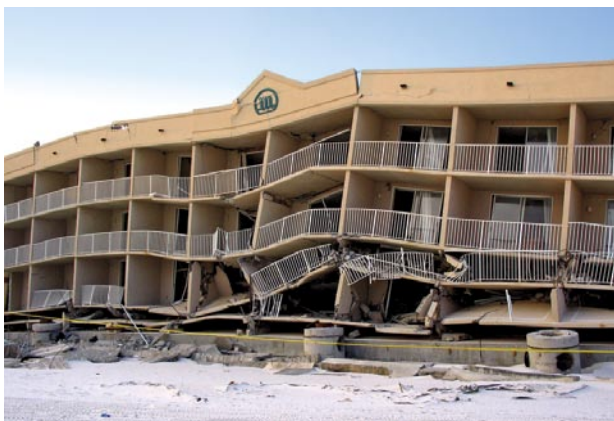
A multi-family condominium collapsed after Hurricane Ivan due to erosion of supporting soil under the shallow foundation.
