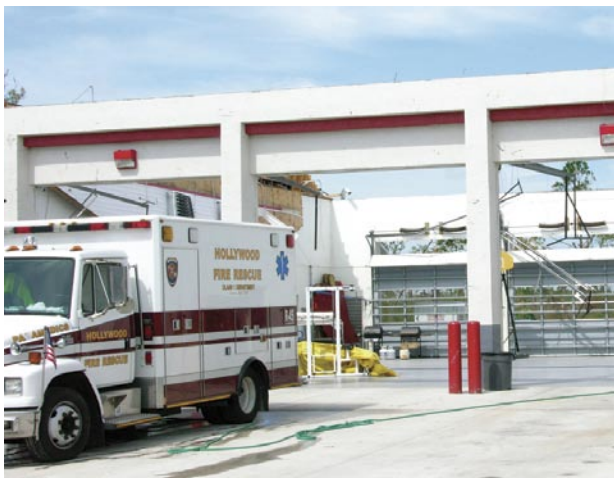
Failure of three of six new doors on a fire station in Charlotte County resulted in the loss of the entire roof structure over the apparatus bay during Hurricane Charley.
