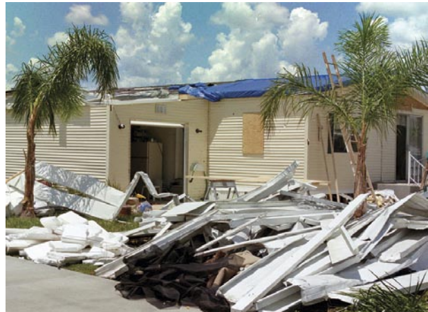
Manufactured housing that had structural damage resulting from accessory structure failure.
